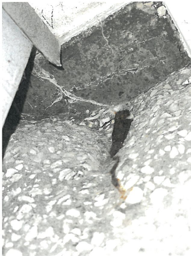
Figure 3: Close up of Exposed Column Reinforcement with Concrete Spall Removed
