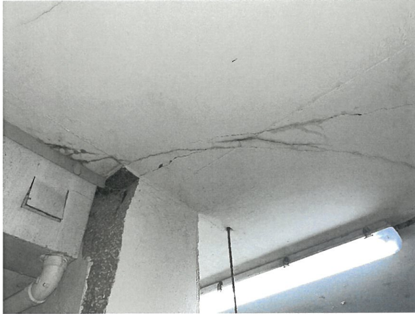
Figure 2: PAA-23 Concrete Column and Slab near Expansion Joint Observed to be Cracked/Spalled
